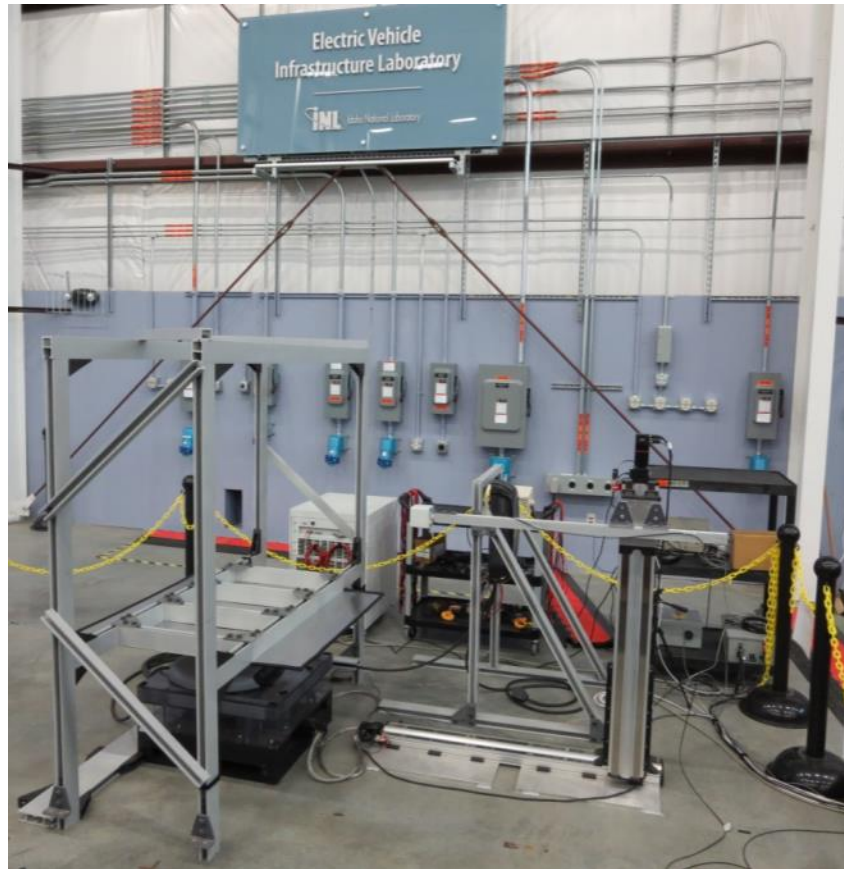
Figure V-1: Bench testing conducted on eight wireless charging systems to support SAE J2954 codes and standards development.
