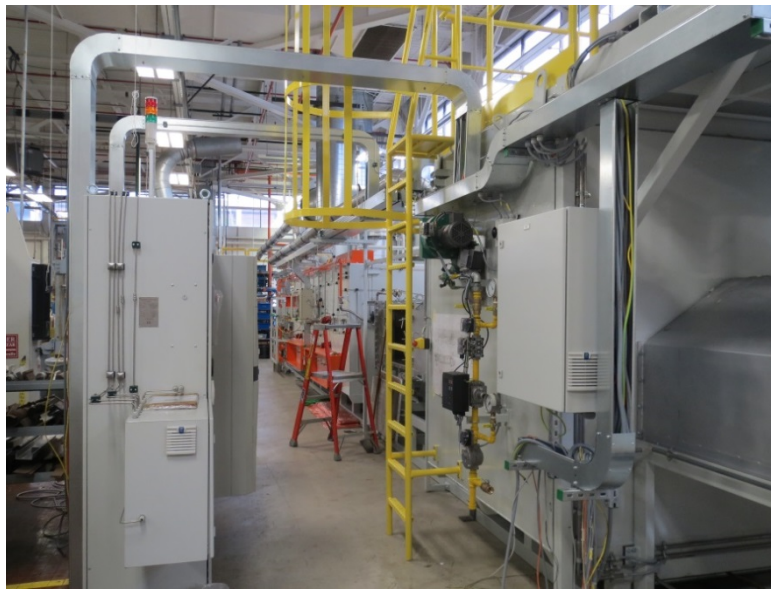
Figure II-75: Controlled atmosphere braze furnace installed in MAHLE Lockport facility
