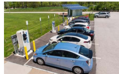
Figure V-17: PEV-EVSE interoperability testbed
