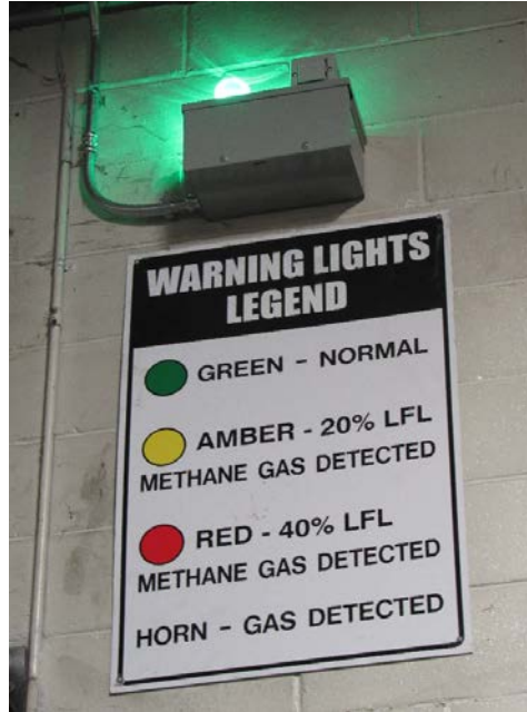
Figure I.18.1: A typical alarm system indicator (Clean Energy Fuels)
