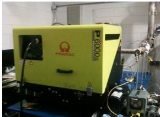
Figure 8. Picture of the stationary generator.
