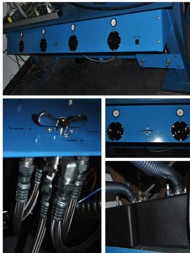
Figure 3. Auxiliary fueling system and manifold panel.
