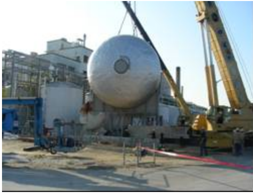
Figure II - 74: FutureFuel – Xylene Tanks-1.
