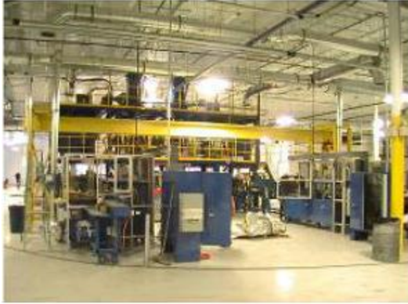
Figure II - 19: Automated Spiral Wound Plate Manufacturing Line in New Advanced AGM Battery Area in Bristol, Tennessee Exide Plant.
