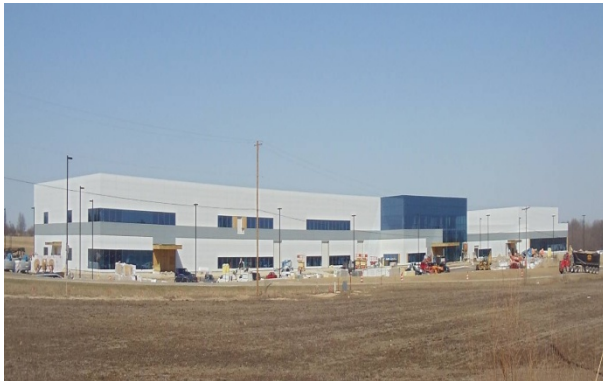
Figure II - 26: LG Chem, MI, Production Facility – Street View – Front of Main Building (1st Qtr. 2011).
