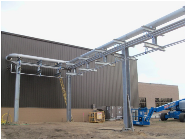
Figure II - 3: Construction included the upfit of an existing building for Li-ion battery production, including the construction of new outbuildings to house equipment and materials.
