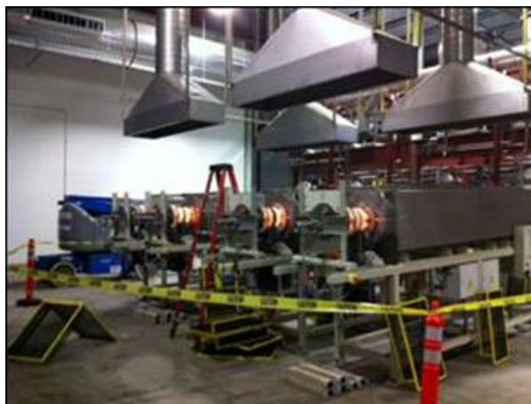
Figure II - 66: Kiln Reactor Commissioning.
