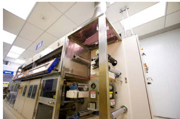
Figure II - 6: Pilot scale equipment installed in controlled environments support the mass production programs.
