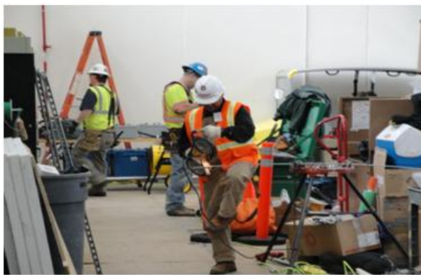
Figure II - 116: TTF Laboratory Chilled Water and Electrical Installation.
