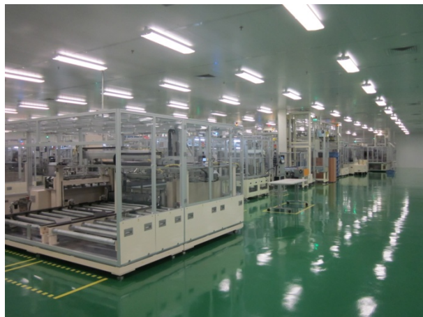
Figure II - 30: LG Chem, MI, Production Facility – Formation Area Equipment.
