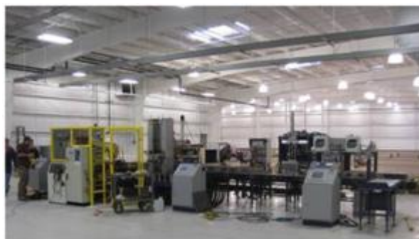
Figure II - 11: New State-of-the-Art AGM Battery Assembly Operation in Columbus, Georgia Exide Battery Plant.
