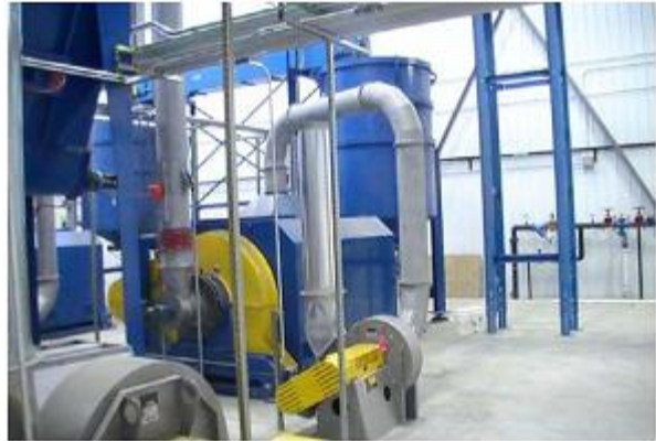
Figure II - 17: New High Purity Lead Oxide Manufacturing Operation in the new AGM area in the Bristol, Tennessee Exide Battery Plant.
