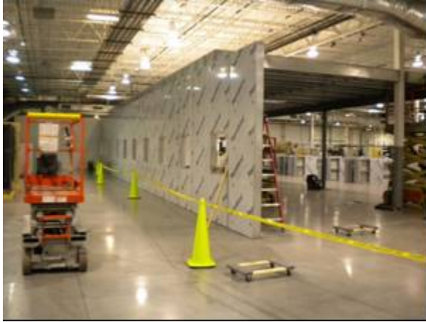
Figure II - 34: EnerDel Lithium-ion Cell Production and Battery Pack Assembly – Dry-room Construction – Hague Rd.
