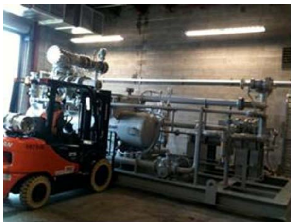
Figure II - 68: Refrigeration Compressor Insulation.
