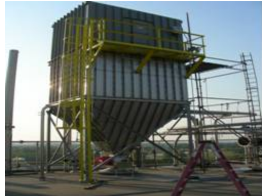
Figure II - 77: FutureFuel – Dryer Baghouse-2.
