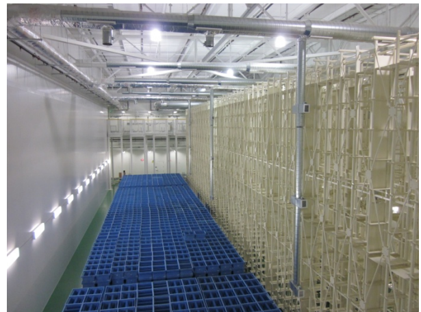
Figure II - 29: LG Chem, MI, Production Facility – Pre-Aging Area Equipment.
