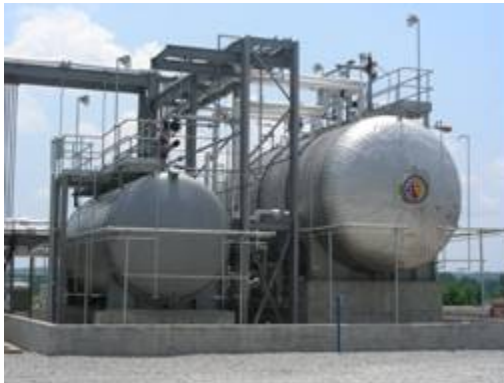
Figure II - 75: FutureFuel – Xylene Tanks-2.
