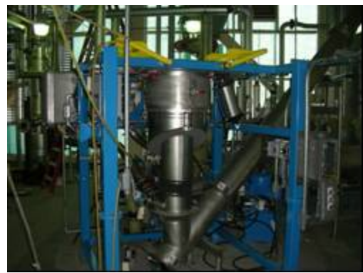
Figure II - 78: FutureFuel – Pitch Loading Hopper.
