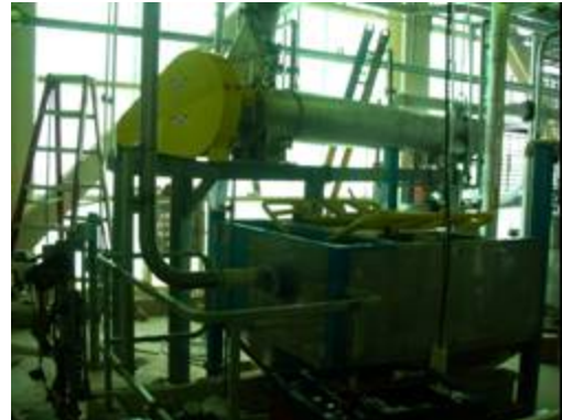
Figure II - 79: FutureFuel – Coke Loading Hopper.
