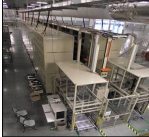
Figure II - 37: EnerDel Lithium-ion Cell Production and Battery Pack Assembly – Cell Formation Equipment – Mt. Comfort.
