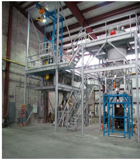
Figure II - 84: Pyrotek Production Facility Project – Equipment.
