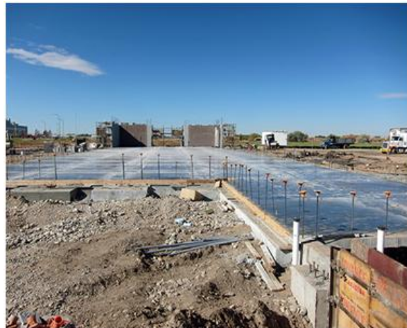
Figure II - 112: Long view of the 10,000 sq. ft. foundation and start of wall construction process in Sept. 2011.
