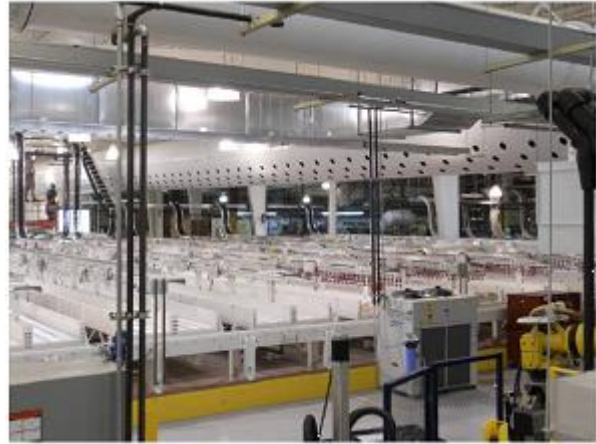
Figure II - 14: Significant Additional Production Capacity in Battery Formation Department – Columbus, Georgia Exide Battery Plant.
