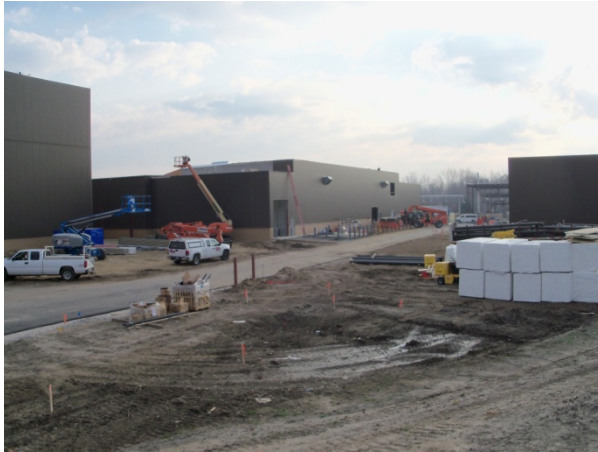
Figure II - 2: Michigan Li-ion battery plant during construction – 1000 construction workers were employed in the construction of our Michigan plant.
