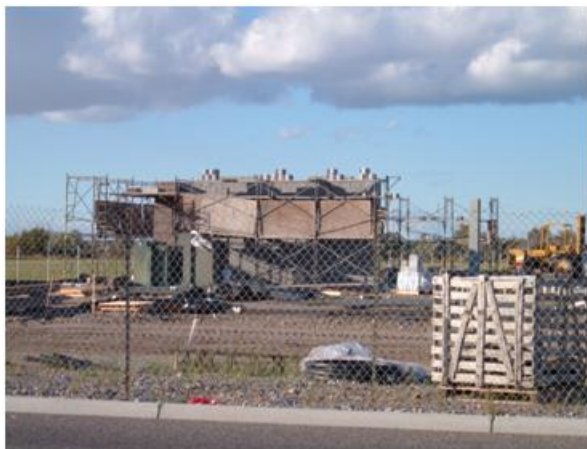
Figure II - 111: Street view of building under construction, new INL High Energy Testing Facility construction began in Aug.of 2011.
