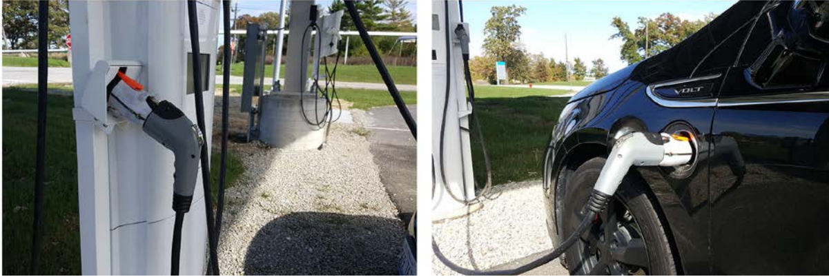
Figure V.1.2 - ANL SCA locked to a public EVSE and connected to a GM Volt while charging (Source: ANL)
