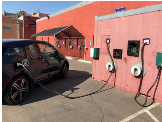
Figure III.6.3 - A 2014 BMW i3 BEV DC fast charging using the StAR unit (enclosed in red chamber) at Intertek in Phoenix, Arizona/Intertek
