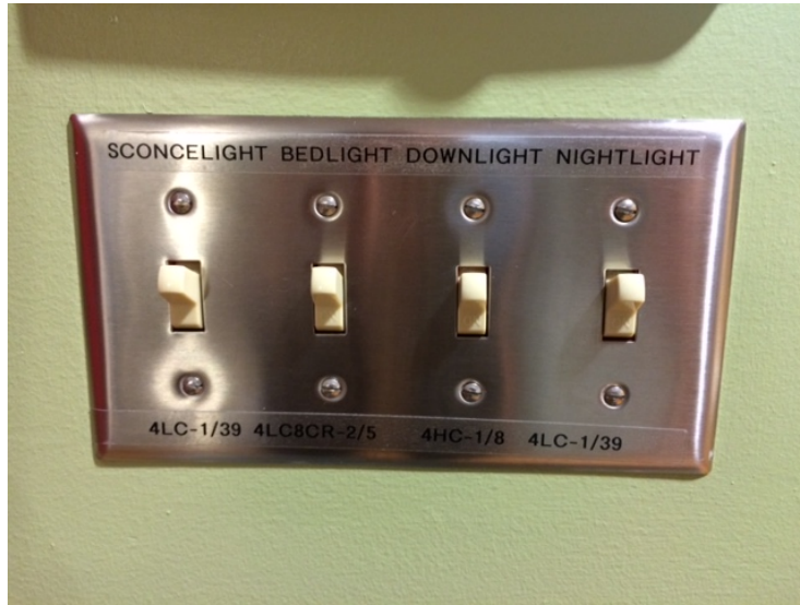
Figure A5: Hospital B wall controller located near the entry door.
