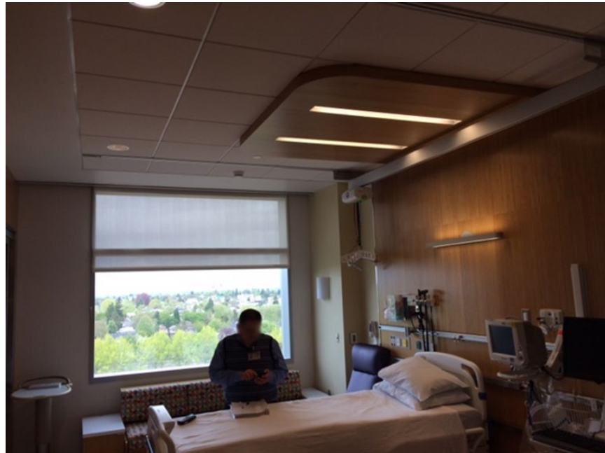
Figure A7: Hospital D patient room showing the recessed round downlight luminaires for general room lighting, the recessed linear luminaires over the bed, the wall-mounted linear luminaire for patient reading, and the wall sconce luminaire in the guest area.
