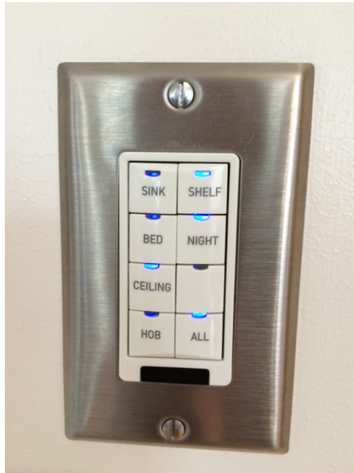
Figure A9: Hospital D patient room push-button lighting controller. HOB refers to the “head of bed” wall-mounted luminaire while “BED” refers to the recessed ceiling lighting over the bed. “CEILING” refers to the recessed downlight luminaires providing general room lighting.
