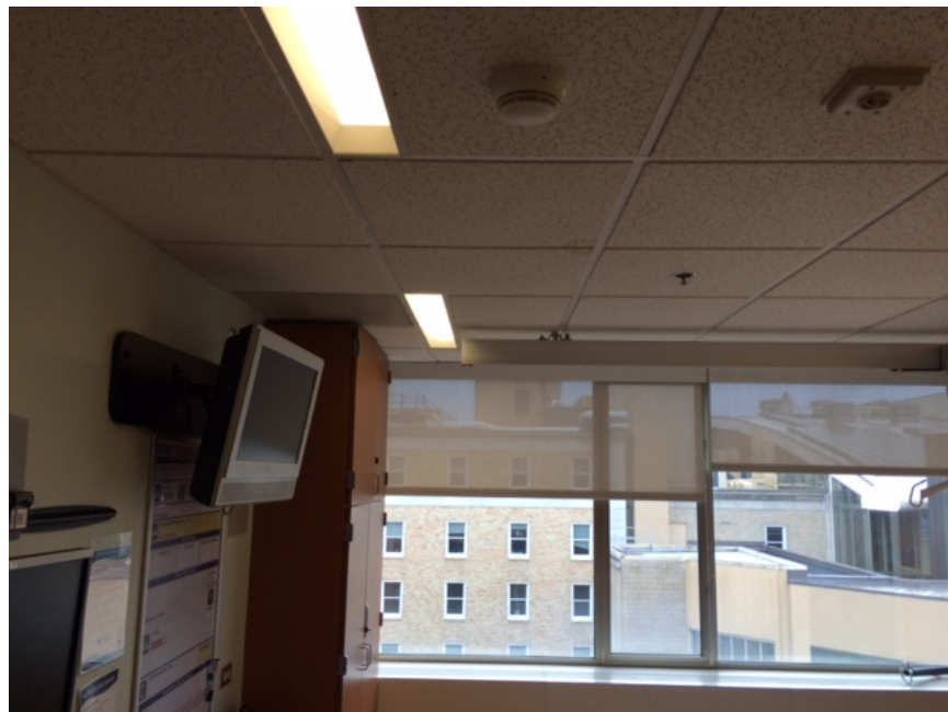
Figure A2: Hospital A patient room showing the recessed linear luminaires providing general room lighting.
