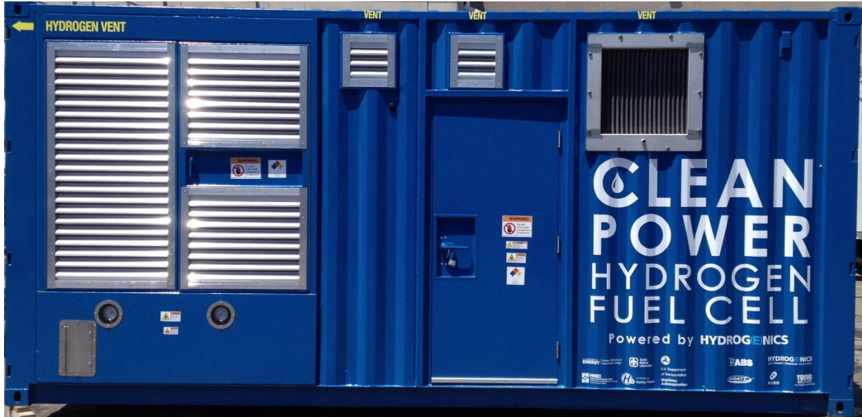
Figure 22: Yellow markings above vents indicate openings not to be blocked.
