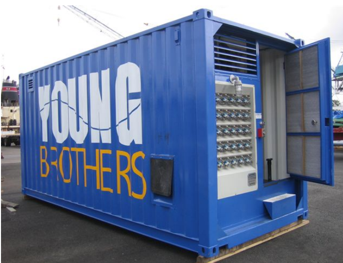
Traditional maritime diesel generator deployed at Port of Honolulu by Young Brothers, Ltd. Photo courtesy of Young Brothers, Ltd.
