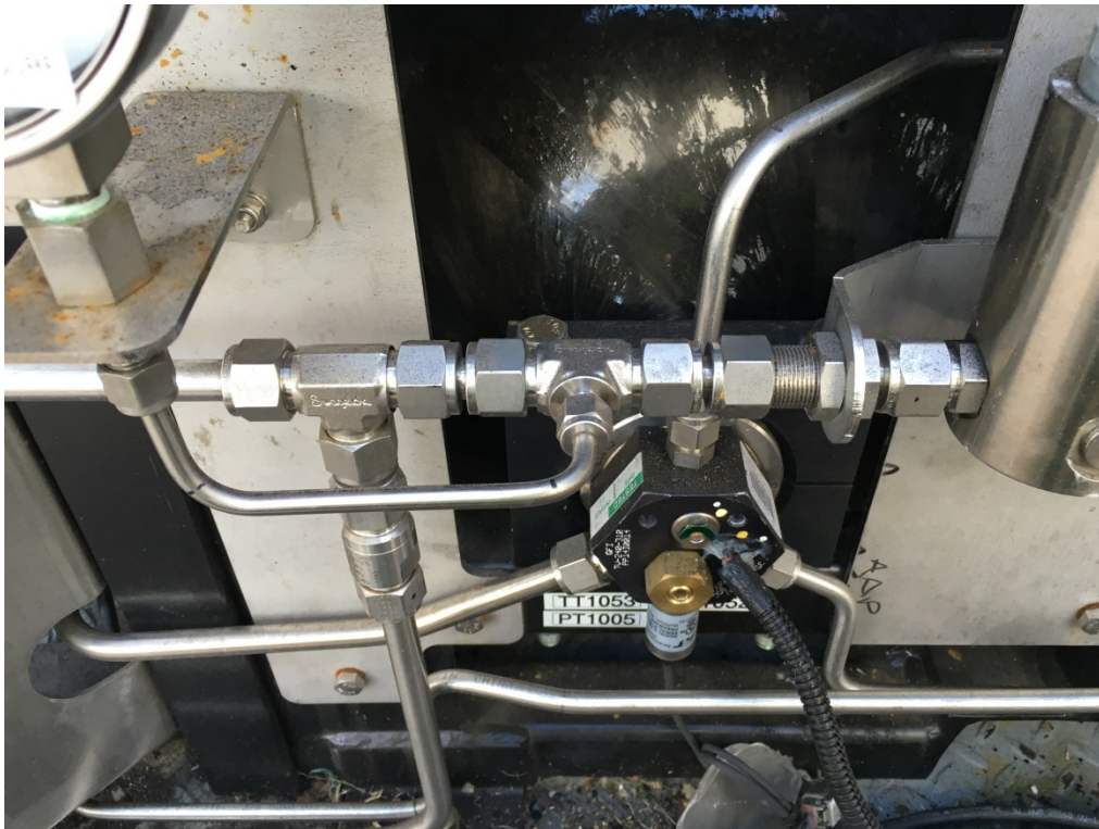
Figure 62: Some of the stainless steel piping inspected for corrosion after 9 months of deployment. Very little corrosion on the piping was observed.
