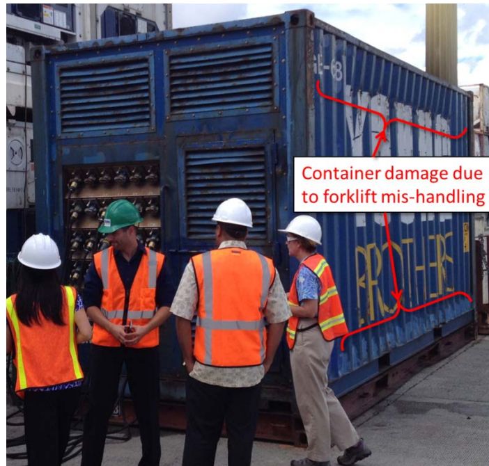
Figure 20: This existing diesel generator showed evidence of damage because of forklift mis-handling. Damage can occur by impacting the forklift’s load carriage or backrest extension, or by impacting the edge of an adjacent container when lowered into place. Damage can also occur if an adjacent container being placed impacts the generator.
