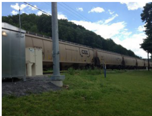
Plug Power fuel cell at railway site
