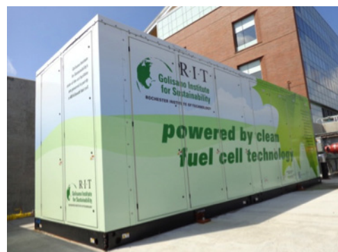
400 kW fuel cell at Rochester Institute of Technology
