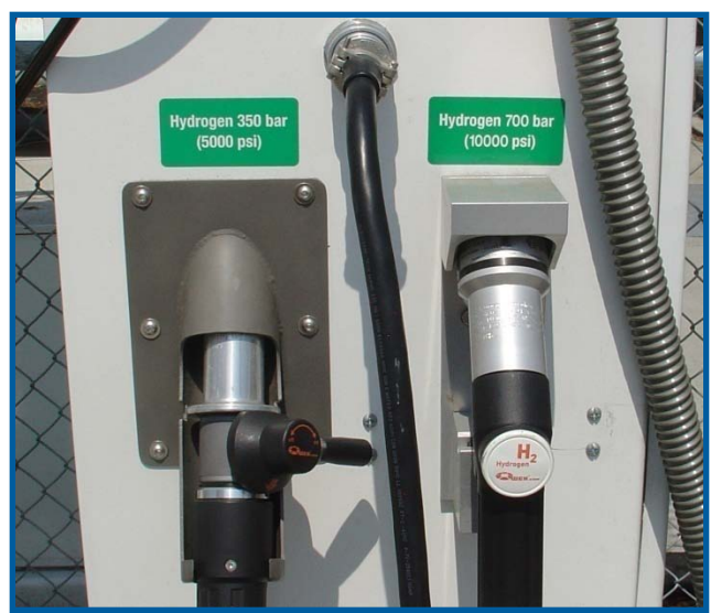
Burbank, CA station. Photo: NREL
