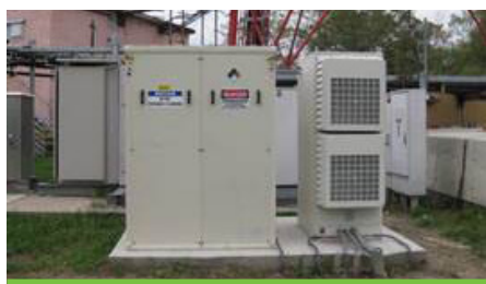
Sprint uses fuel cells to provide backup power to their cell phone towers.
