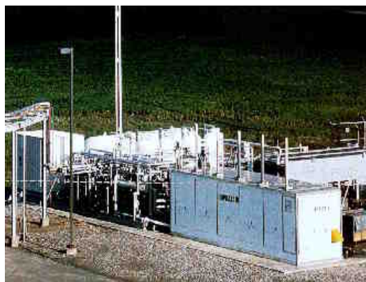
Figure 3. Praxair HGS On-Site Supply System (Seymour, Indiana)
