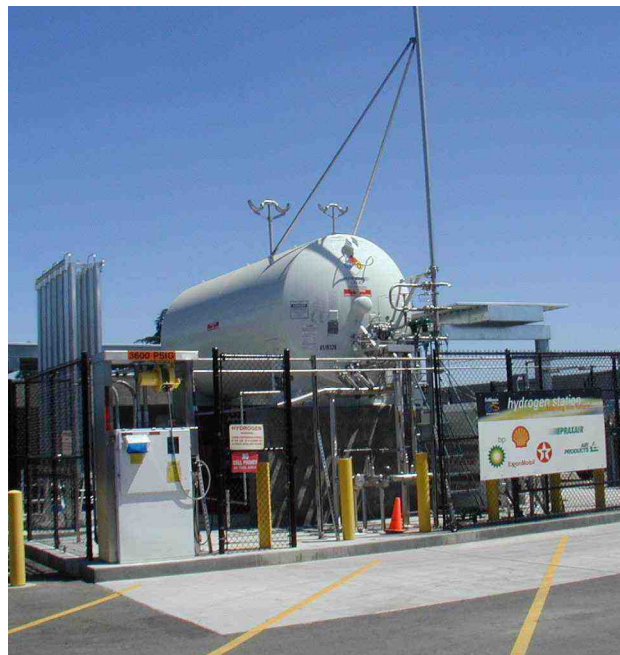
Figure 3. CaFCP Hydrogen Refueling Station
