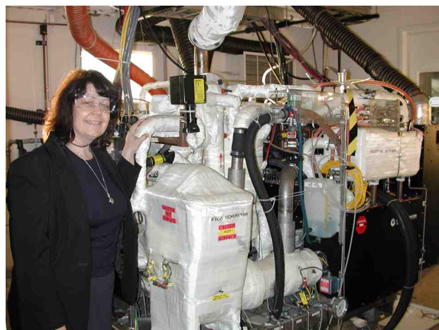
Figure 4. 50 kW power plant installed in ANL test facility
