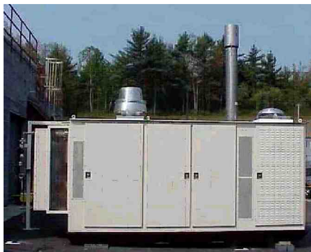
Figure 2. 50 kW Fuel Cell Power Plant
