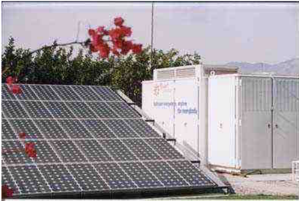
Figure 2. P3-1A Fuel Appliance at SunLine Transit, 1000 Palms, California
