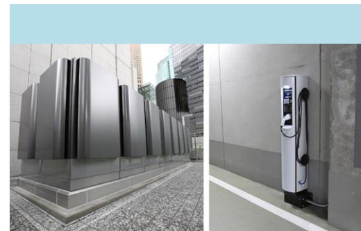
Tokyo Shiodome - Bloom Energy Server (left) supplies power to both the facility and the building's EV charging stations (right)
