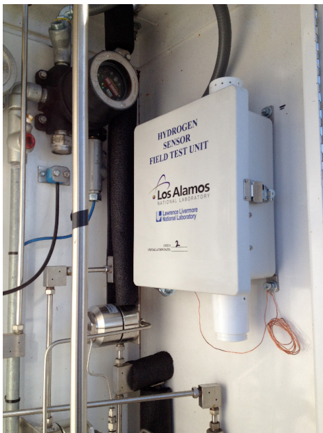
Packaged Electrochemical H 2 Safety Sensor Deployed for Field Trials Testing
