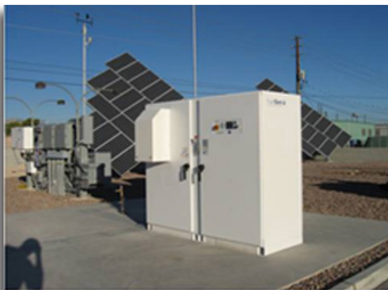
FuelGen Station in Las Vegas, NV
