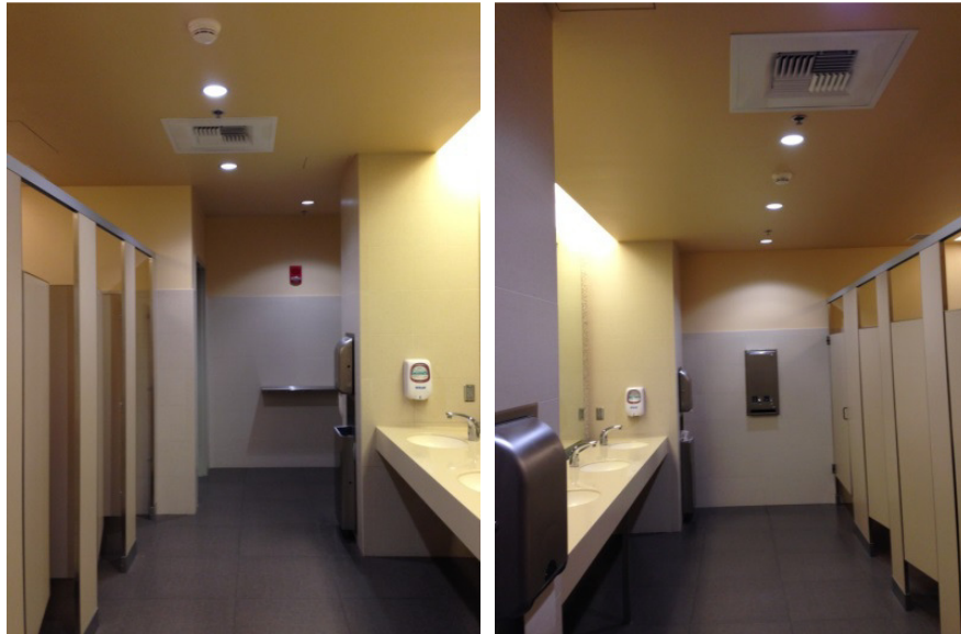
Figure 3. The CFL downlights in the restrooms were re-lamped with LED replacement lamps. The photos show the ground floor ladies' restroom after the LED conversion. Photo credit: PNNL.
