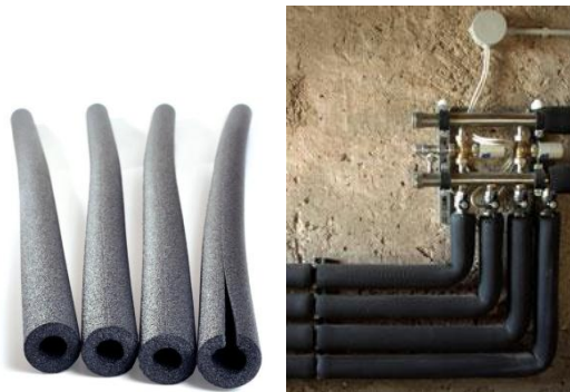
Figure 6-20: Typical Use of Piping Insulation
