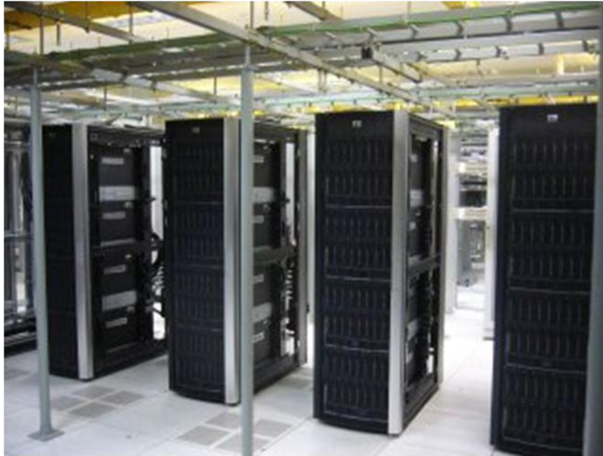
Figure 5-4: Server Racks in a Data Center
