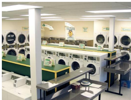
Figure 8-1: Coin-Operated Laundry Featuring Washers and Dryers Of Various Sizes and Configurations.
