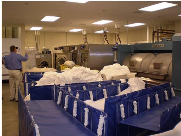
Figure 8-3: On- Premise Laundry Facility Featuring Large-Capacity Washing and Drying Equipment
