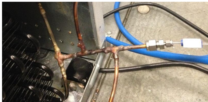
Fig. 2.8: Instream thermocouple for refrigerant side temperature measurement
