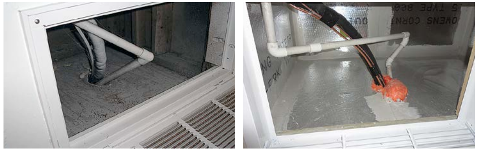
Pre-retrofit: Typical unsealed return plenum (left). Post-retrofit: Return plenum edges and seams are sealed, preventing return air from non-interior spaces, saves energy, and improves indoor air quality (right).
