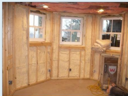
Foundation wall, after installation of all moisture and thermal management layers. The space is now ready for finishes.
