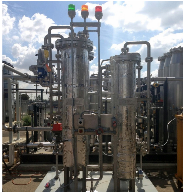
Sulfur polishing skid installed at the South Area Transfer Station (SATS) in Sacramento, CA. Photo credit TDA Research Inc.
