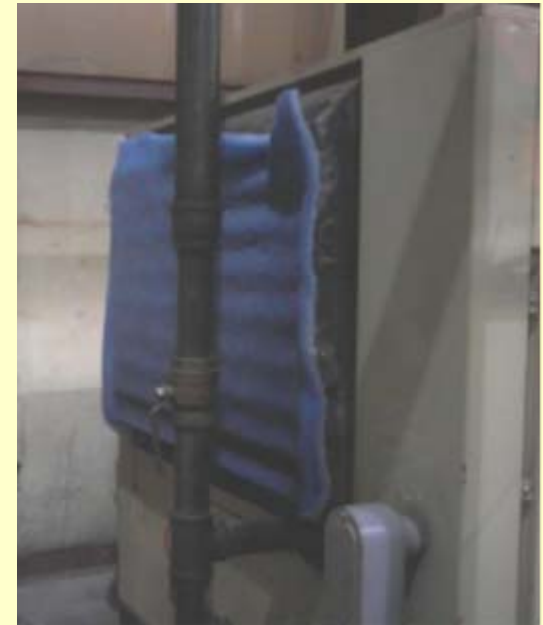
Air intake inside
