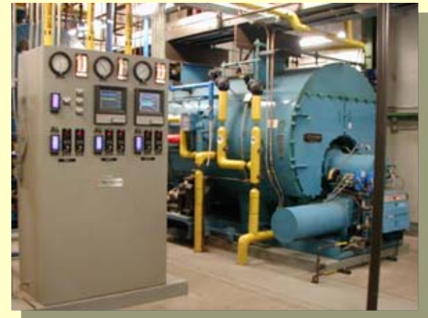
Fire tube boiler with O2 Trim system.
