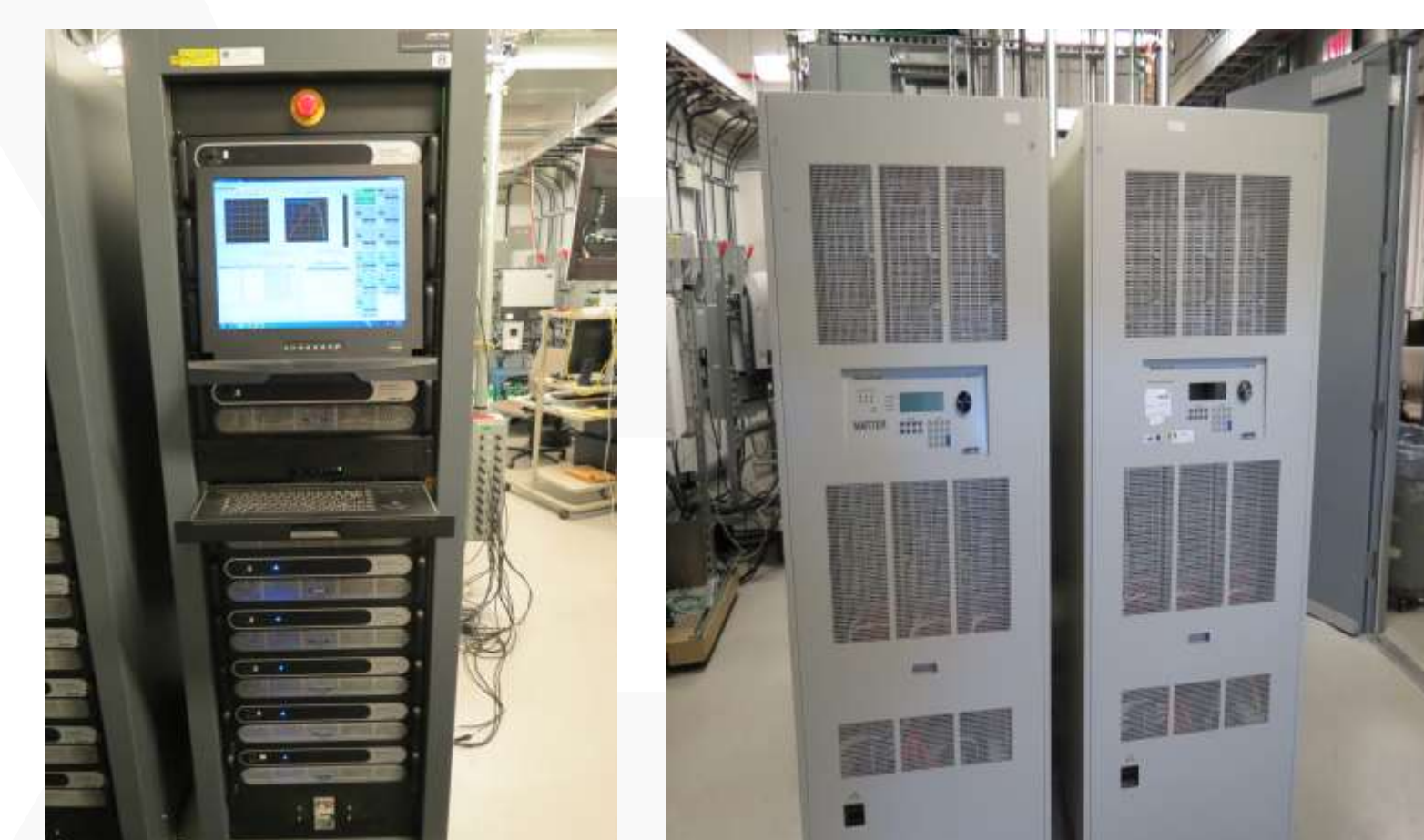
Lab equipment at Sandia for evaluating conformance test procedures: Amtek 100kW PV simulator (left); AC simulator (right)
