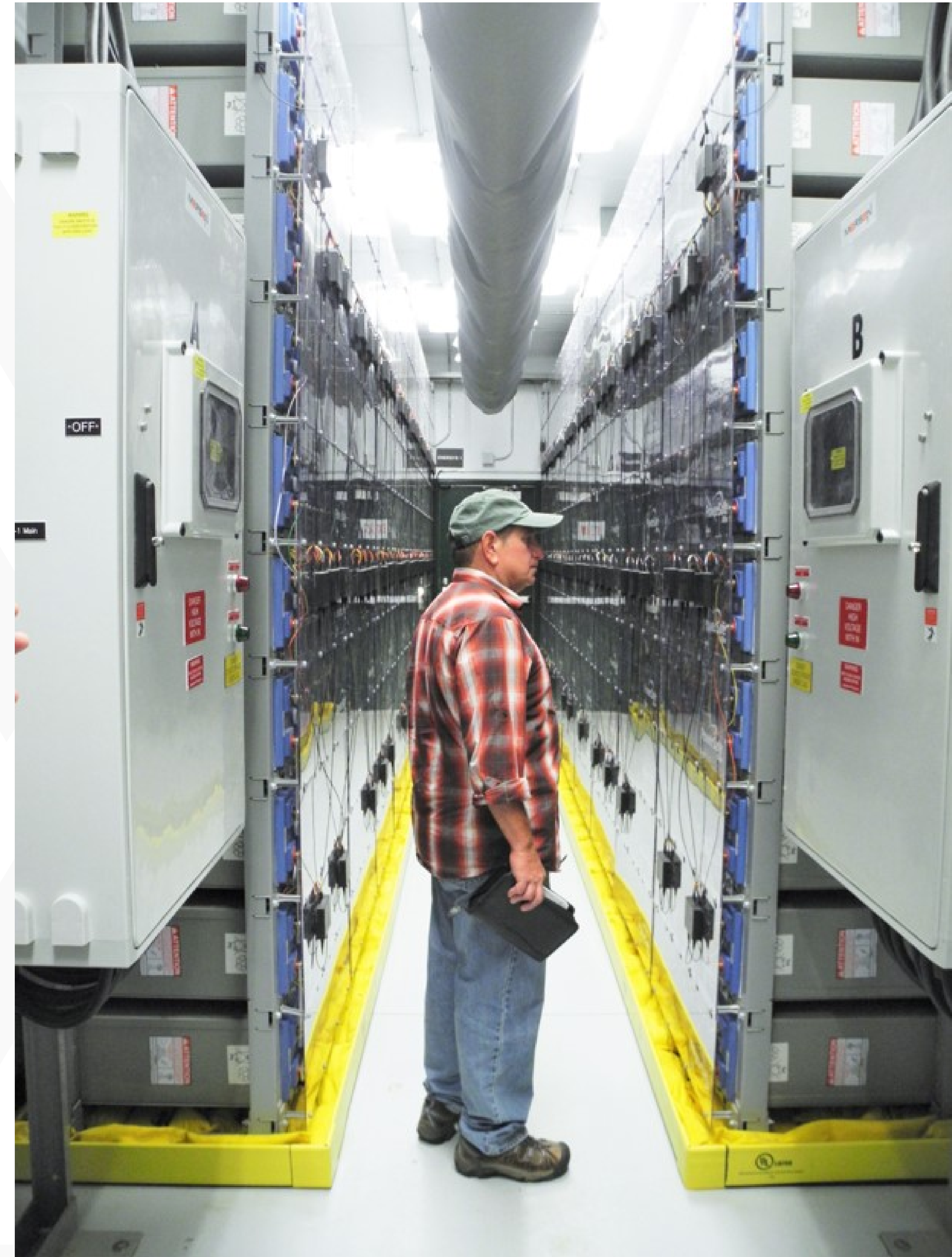
Principal Investigator, Dan Borneo, with Sandia National Lab, views a battery system.
